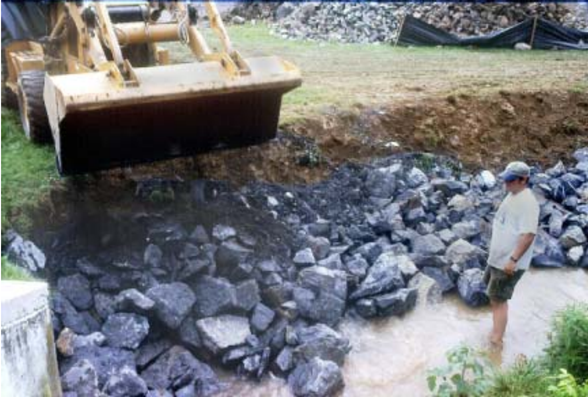
Figure 6. The placement of “hard structure” was appropriate along this stream bank due to the proximity of the foot bridge. Sawtooth deflectors are designed to direct the flow of water away from the stream bank and toward the center of the stream channel.
