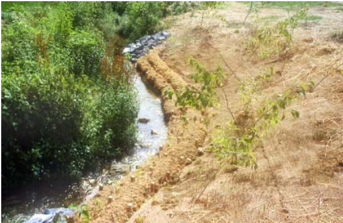
Figure 14. Natural materials were incorporated into the restoration design where appropriate. The use of coconut coir logs allowed for vegetated toe stabilization that would mimic the natural contours of the stream.
