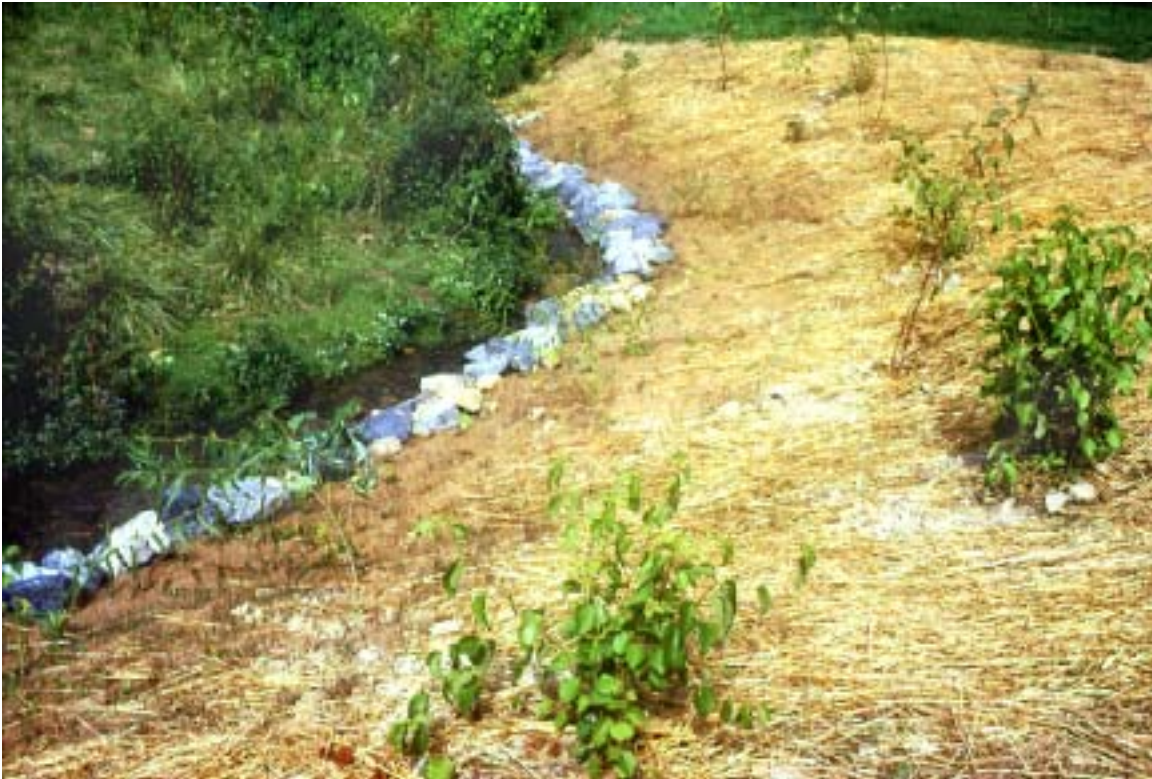
Figure 17. Modest quantities of stone were used along certain banks that required less aggressive stabilization techniques.
