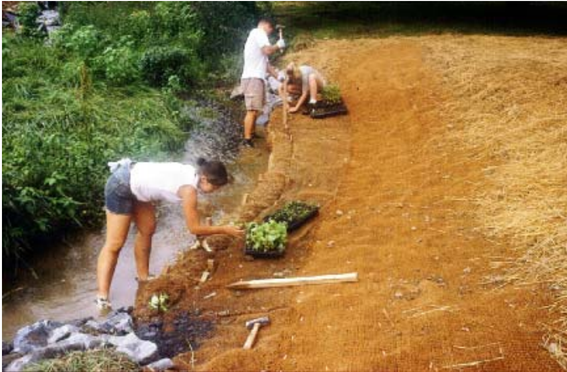
Figure 13. Cooperation and ingenuity allowed for the efficient implementation and completion of this project. In this photo, Wildlands Conservancy staff drive oak stakes into biodegradable coconut logs for the insertion of herbaceous plugs.
