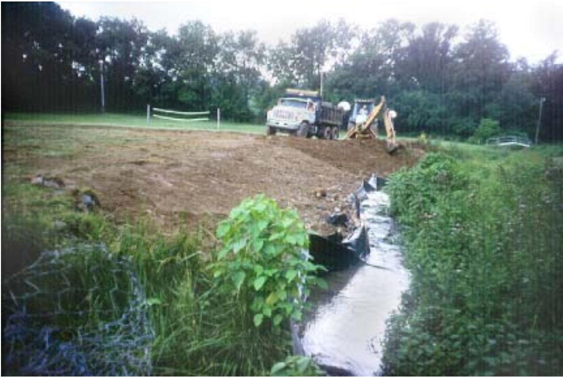
Figure 3. An approximate 3:1 grade was applied to this length of bank following gabion basket removal. Silt fencing was used to minimize siltation and adhere to erosion and sedimentation control practices.
