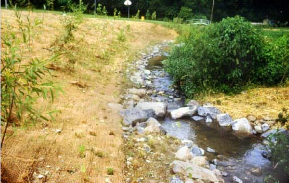
Figure 9. Grading stream banks allows streams access to their floodplains where they can dissipate their energy. Floodplain access and grade control is important in reducing water velocity and stream bank erosion.
