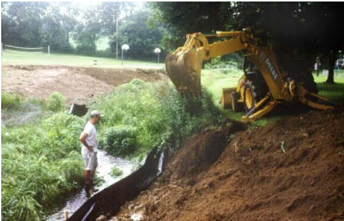
Figure 12. Communication with equipment operators is essential in assuring that restoration techniques are implemented to design specifications.
