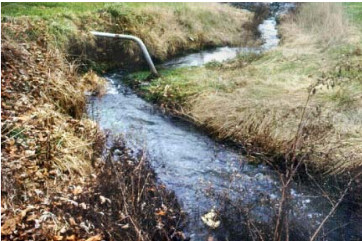
Figure 18. This picture illustrates the tendency of the stream to meander in time, thus exposing an electric line that was once buried in the stream bank.
