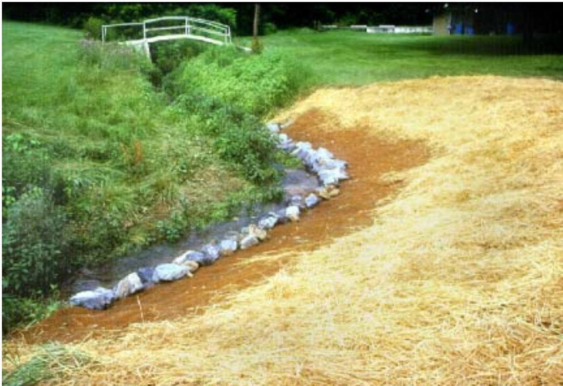
Figure 16. The use of biodegradable erosion control blanket and straw will provide moisture retention for newly planted vegetation.
