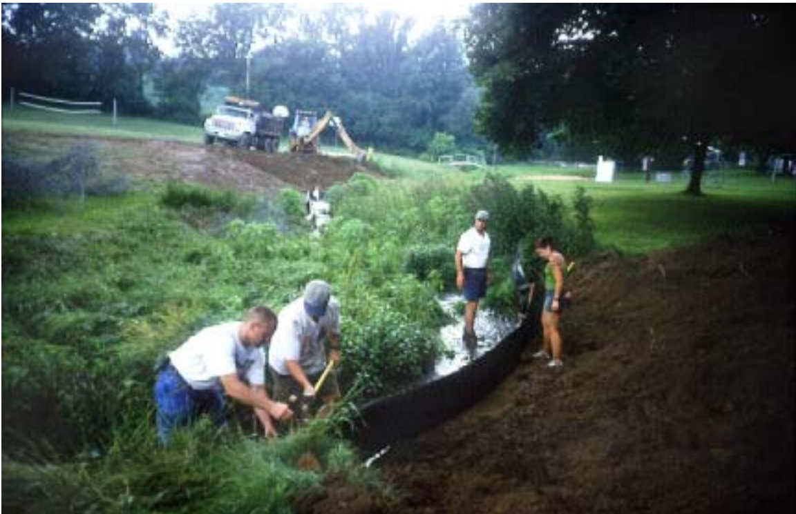
Figure 11. The availability of multiple excavators allowed for simultaneous bank work, which was necessary for the timely completion of this project.
