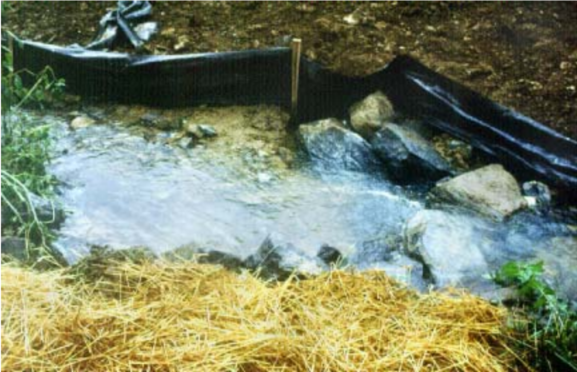
Figure 8. Rock weirs were installed to provide grade control and habitat diversity within a high gradient stream reach dominated by shallow riffles. These devices should have a cumulative effect in reducing water velocities throughout the tributary.
