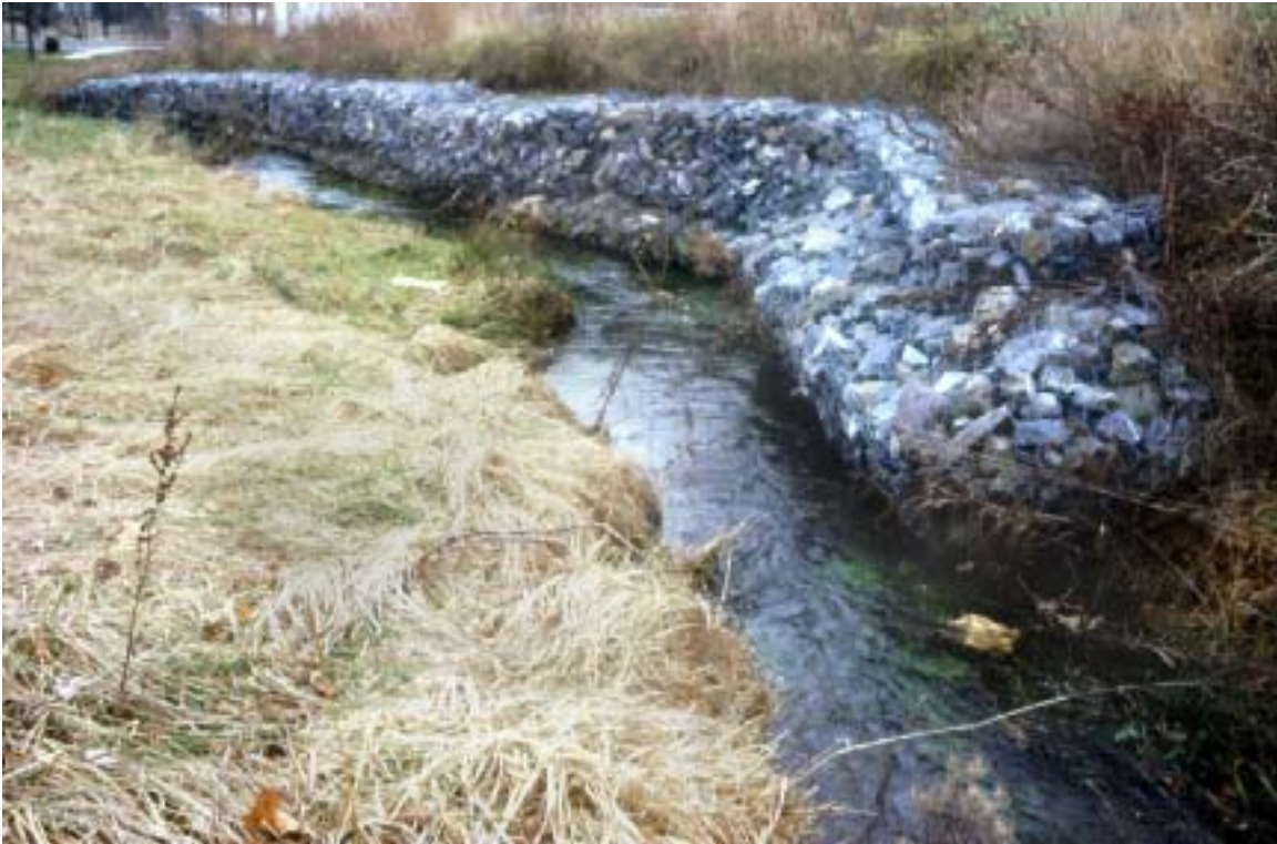
Figure 1. Gabion baskets have channelized a portion of the stream reach within Keystone Park. Stream channelization, urban storm water and a lack of riparian vegetation have impacted this reach by accelerating bank erosion and sedimentation.
