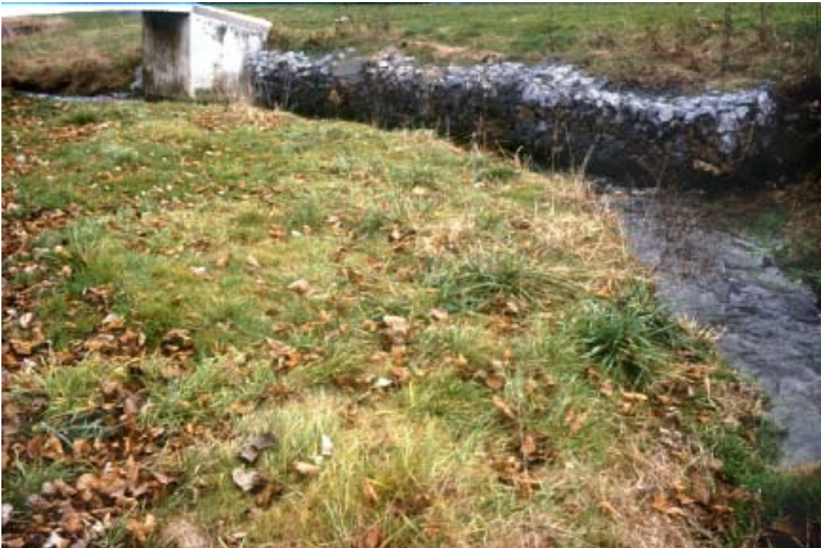
Figure 5. Gabion baskets within the park were structurally failing and offering little opportunity for the establishment of bank vegetation. Before the project was implemented, grass was mowed to the edge of the stream banks.
