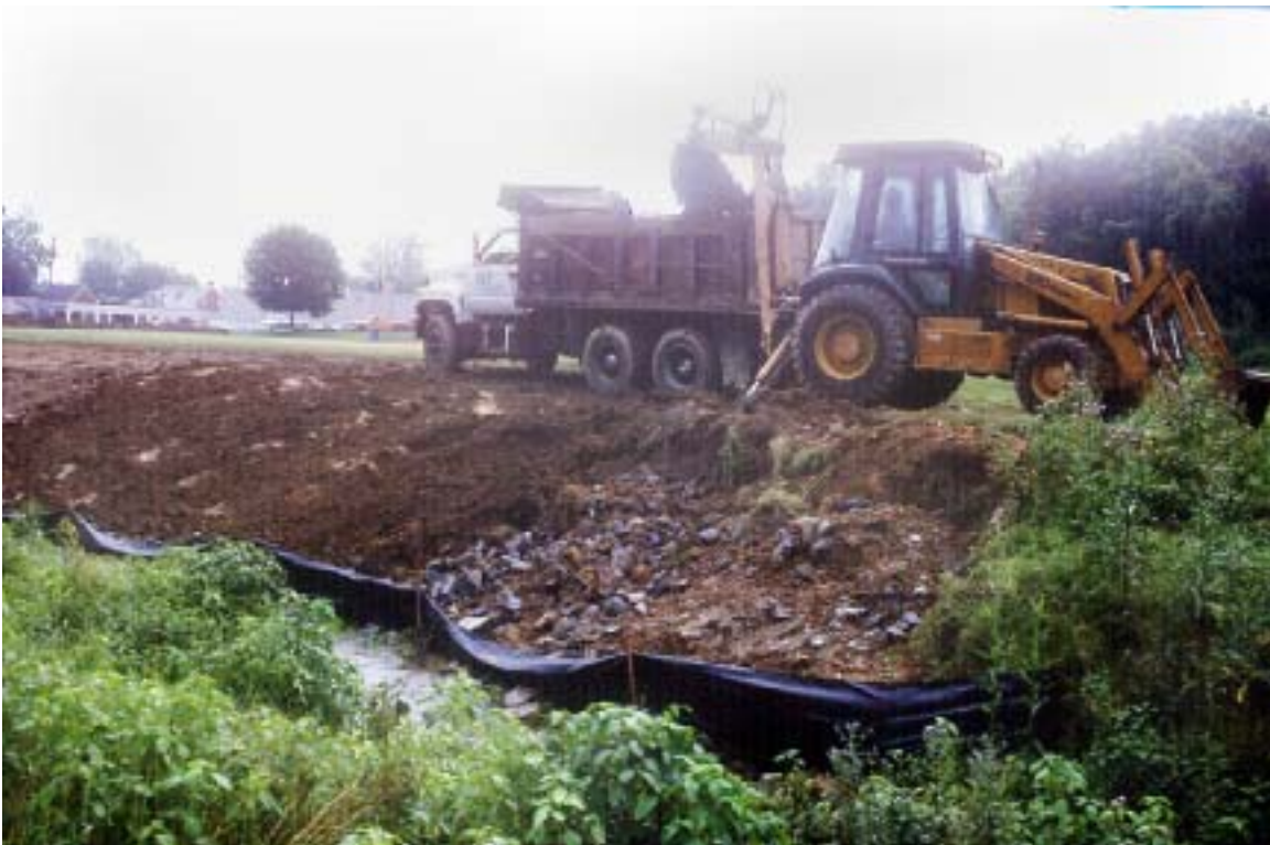
Figure 2. Gabion basket removal. To remove the baskets, a trench was excavated behind the baskets so that they could be pulled away from the channel. This method of removal minimized impacts to the stream. The stone that was contained within the baskets was used to stabilize the toe of this bank after grading was completed.
