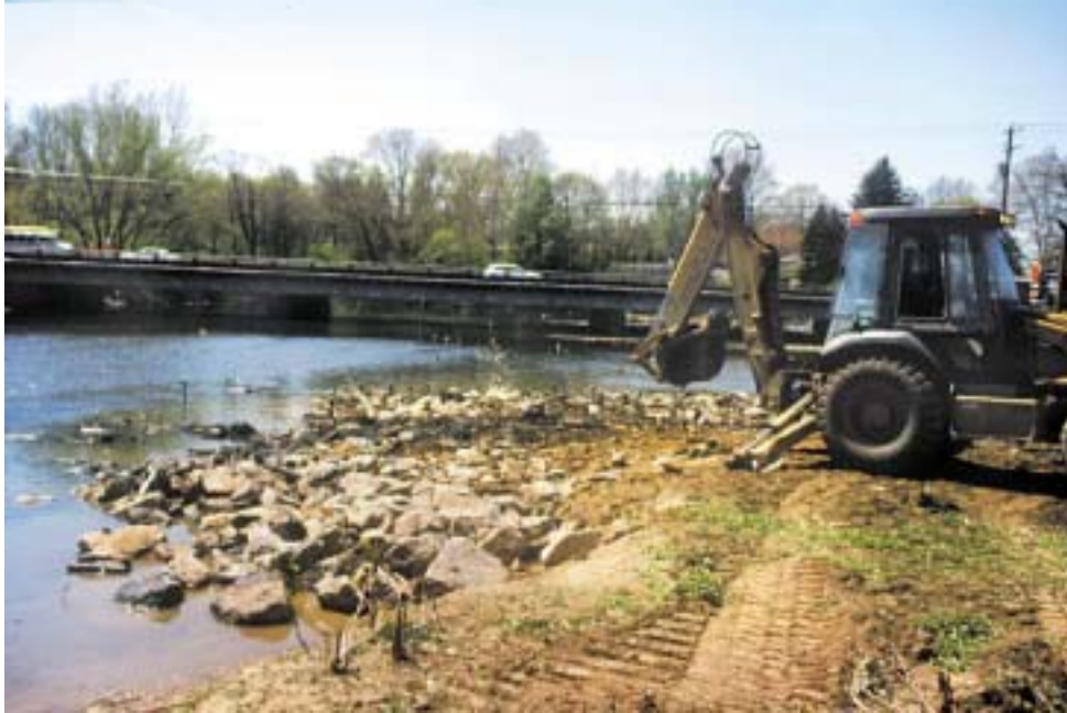
Figure 11. A backhoe was used to construct the stone and saw-tooth deflectors. The deflectors were constructed using mixed sizes of stone, and were dressed with layers of topsoil to provide a medium for the establishment of native trees, shrubs and grasses.
