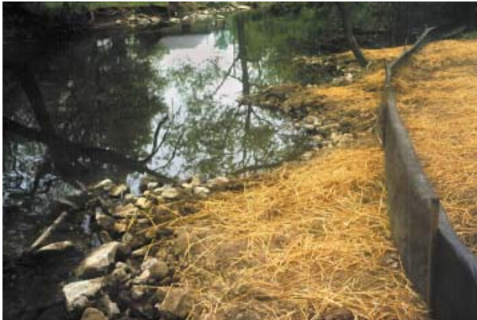
Figure 8. Saw-tooth deflectors were constructed to provide stream bank stabilization and improved aquatic habitat. A layer of topsoil was placed over the deflectors to provide a medium for the establishment of native vegetation.
