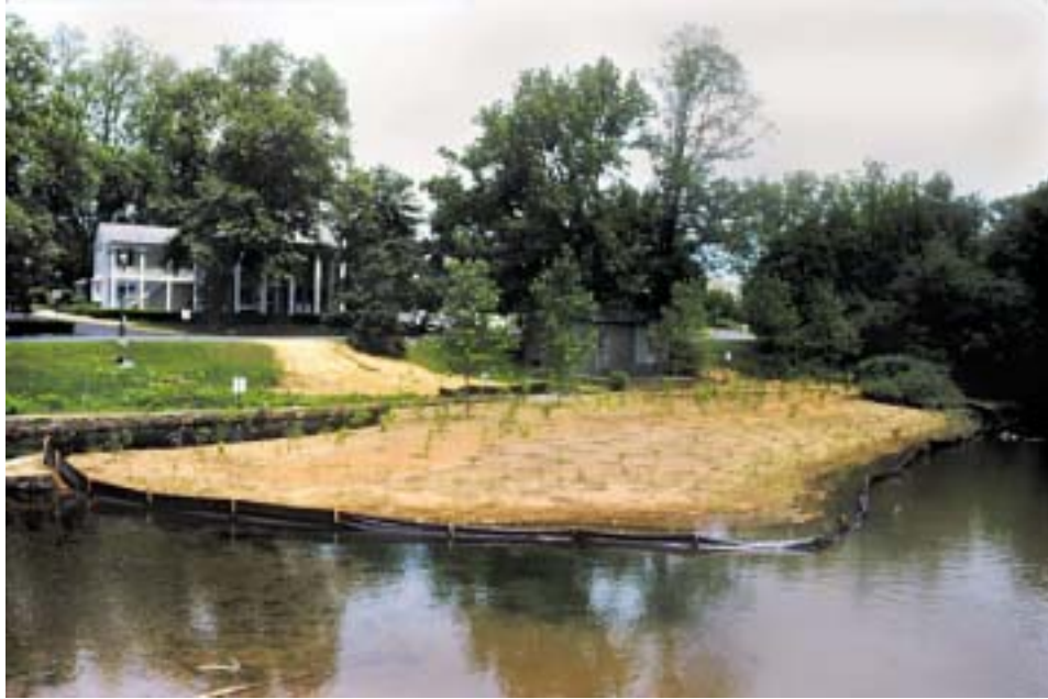
Figure 17. An upstream view of the project site immediately following the construction of stream improvements and the establishment of a riparian buffer.
