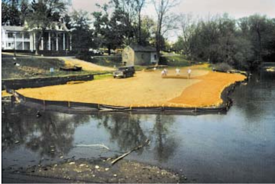
Figure 13. Silt fencing was erected around the perimeter of the deflector to prevent sediment from entering the stream during and prior to construction. Upon completion of the deflector, native wetland, transitional and upland seed mixtures were applied to the soil. Biodegradable coconut blanket and straw mulch was used to provide soil stabilization and to promote vegetative growth.
