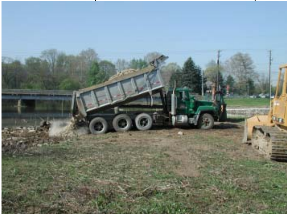
Figure 10. Approximately 600 tons on stone were used to construct the stream improvement devices, which consisted of one stone and three saw-tooth deflectors.
