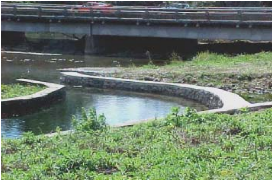
Figure 6. The area immediately behind the wall was back filled with stone and soil to provide a medium for the establishment of native trees, shrubs and grasses.
