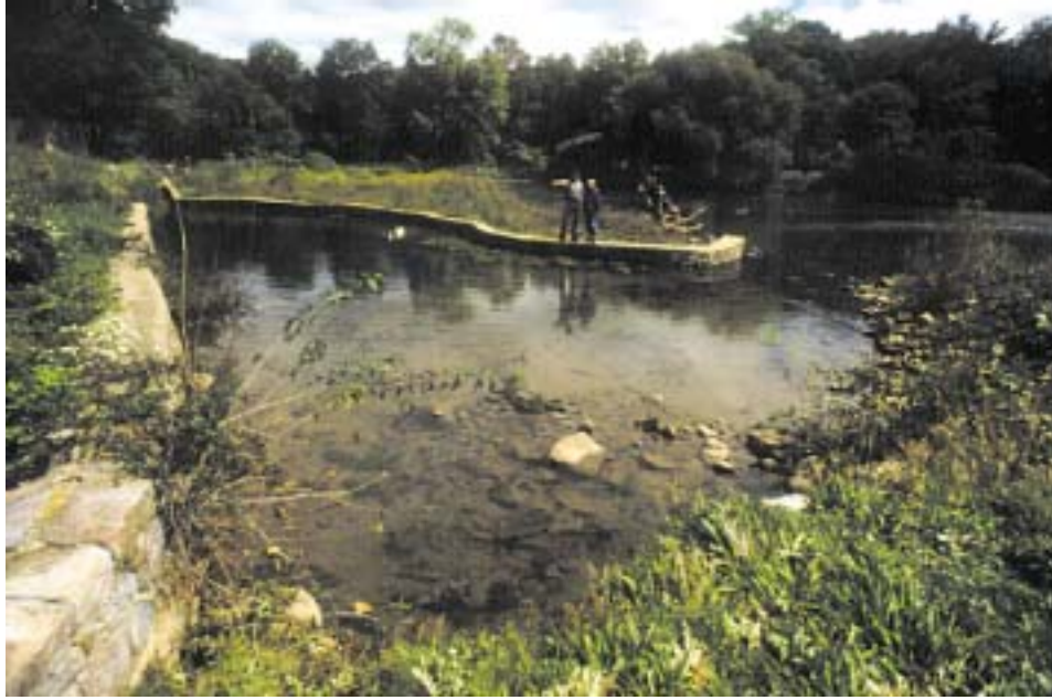
Figure 3. In addition to establishing a riparian buffer and constructing stream improvements, the project included the restoration of a historical spring raceway that empties into the Monocacy Creek. Note the riparian vegetation present after a “no-mow” management style was implemented as a preliminary, short-term recommendation until implementation of the project.
