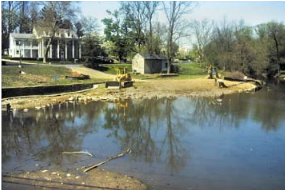
Figure 12. A view looking upstream at the project site from Route 512, after two days of excavation work on the stone deflector had been completed.
