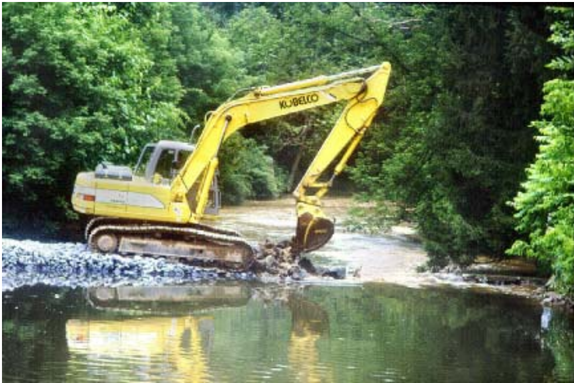
Figure 7. An appropriate rate of water draw down was established by regulating the size of the notch.
