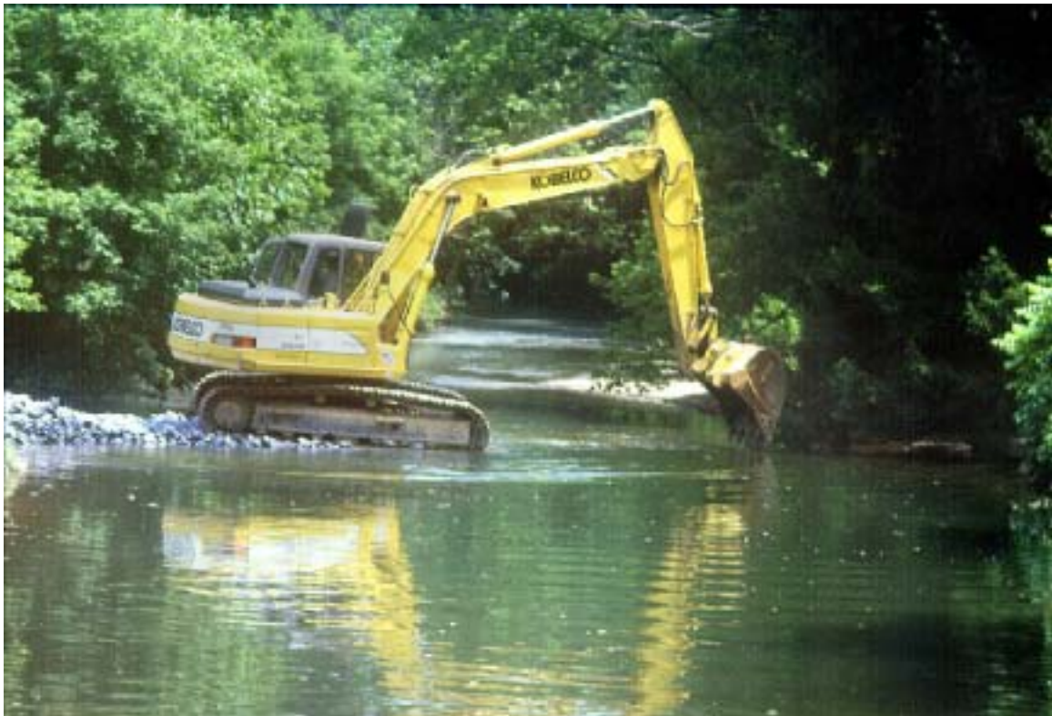
Figure 6. Once the hydraulic jackhammer was used to puncture the dam, the concrete was removed to create a notch in the dam breast on the far bank.
