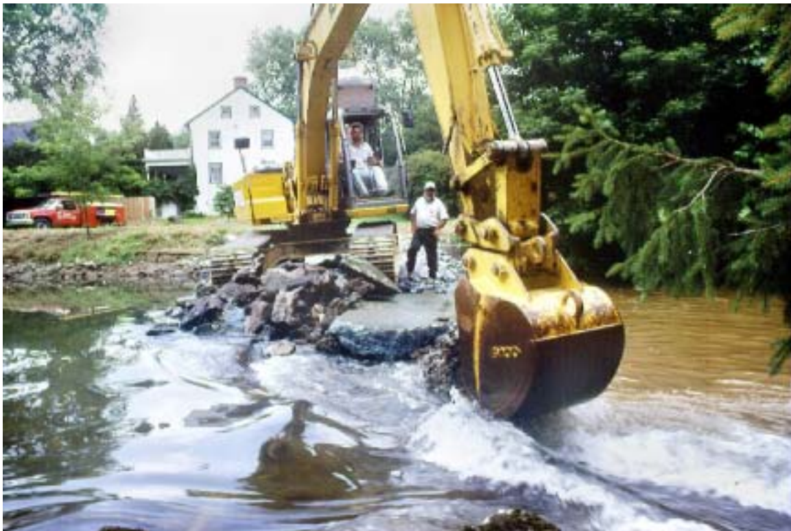
Figure 8. Once the initial dam breach was completed, concrete was continually removed to increase the size of the notch.
