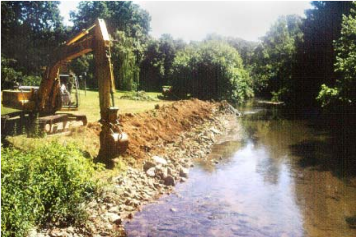
Figure 15. A concrete retaining wall approximately 190 feet in length was removed before creating a grade transition from the top of the bank to the streambed.
