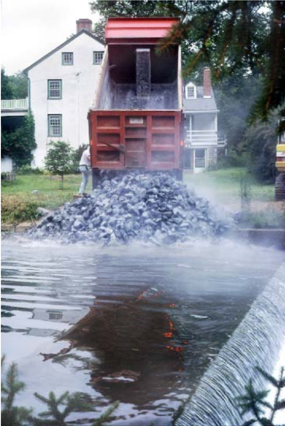
Figure 2. The stone that was used during the project was purchased and delivered from a local limestone quarry. Suitable access to the dam existed along the left streambank (looking downstream).
