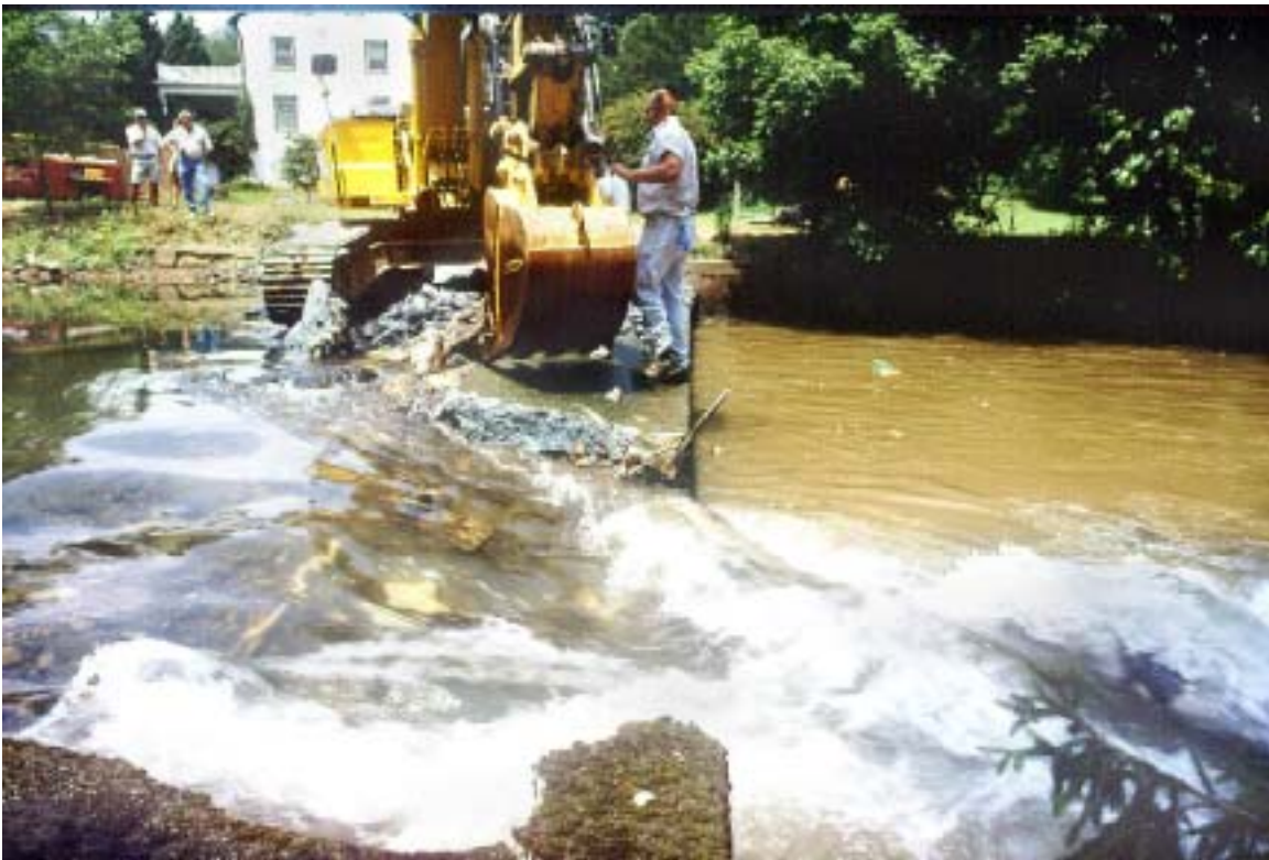
Figure 9. The dam breach excavation was paused periodically to assess the condition of the breach and allow a controlled draw down.
