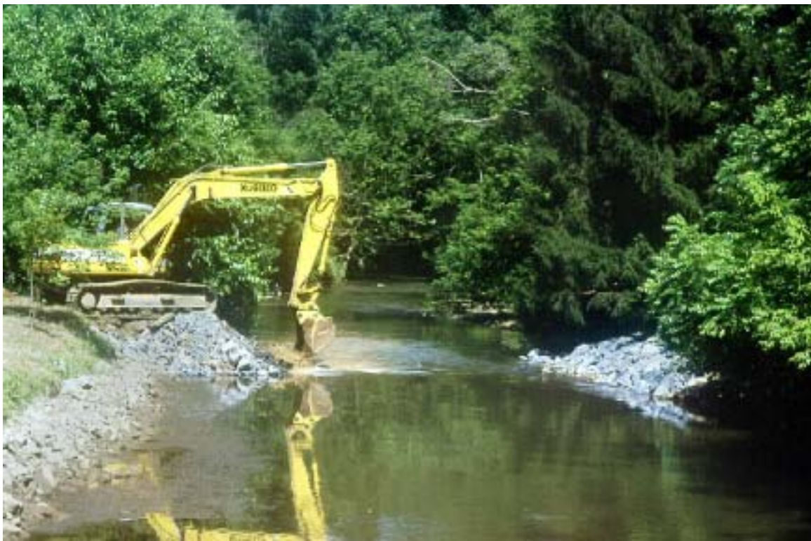
Figure 14. Once the opposite stream bank was stabilized, the remainder of the dam was removed. The stone causeway was then removed and used to provide stone to stabilize the near stream bank.
