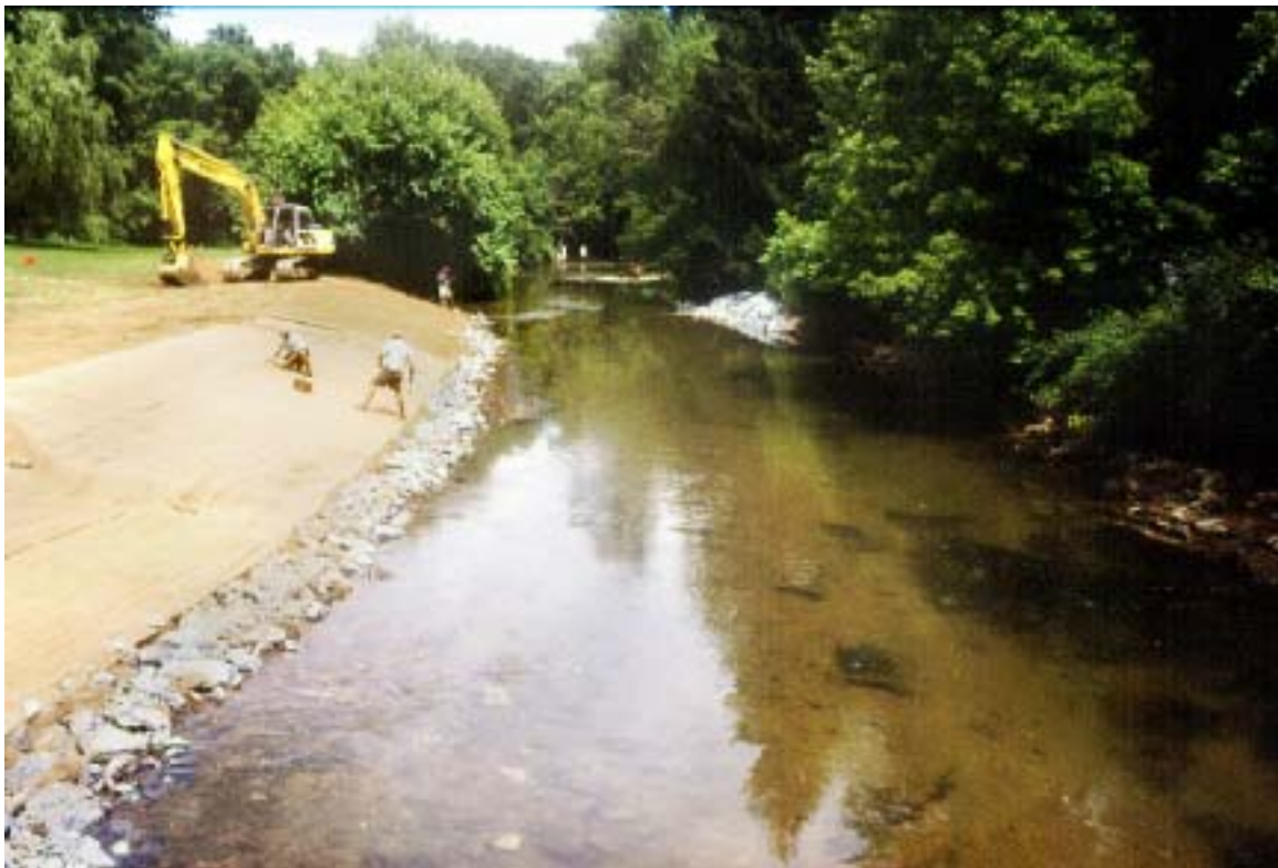
Figure 17. After stream bank grading was completed, stone riprap was placed along the toe of the stream bank to provide bank stability. Two access paths were excavated before applying biodegradable erosion control blanket along the length of stream bank.
