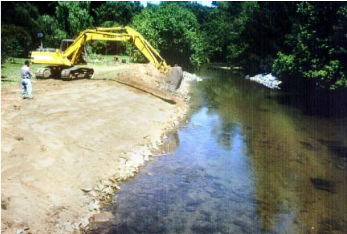
Figure 16. Once the concrete retaining wall was removed, the stream bank was graded to an approximate 3:1 grade. This grade will allow stream bank vegetation to become established. Impacts were minimized during bank grading by drawing soil away from the stream.
