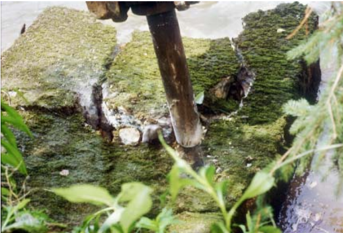
Figure 5. Portions of the concrete dam were broken into pieces that were manageable and easily manipulated.
