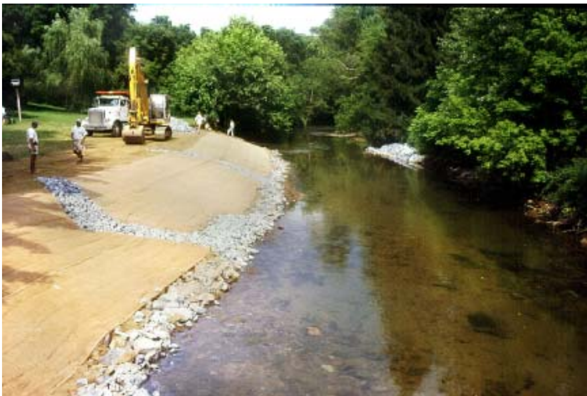
Figure 18. The erosion control blanket was secured to the stream bank using biodegradable stakes. Access paths were installed to provide access for educational groups utilizing the stream corridor.
