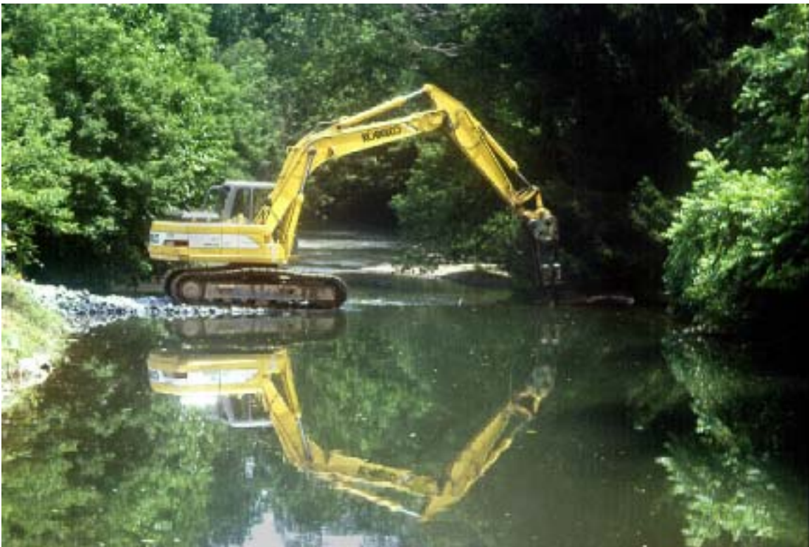
Figure 4. Once equipment access was established, a hydraulic jack-hammer was attached to the track-hoe and used to puncture the dam breast.
