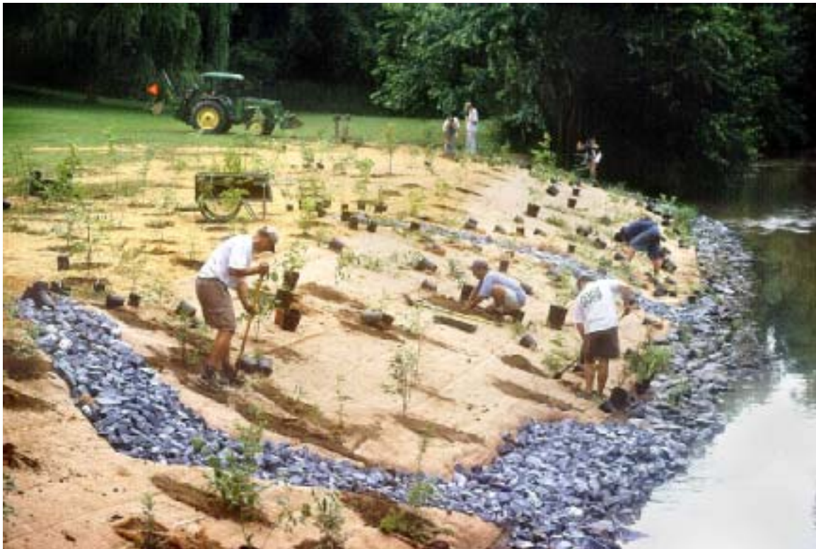
Figure 19. Several varieties of native trees, shrubs and herbaceous material were planted to establish a riparian buffer along this section of the Little Lehigh Creek. This vegetation will minimize soil erosion and provide shade to the stream, maintaining the cool stream temperature essential to fish and macro-invertebrate survival. Stream bank vegetation offers habitat for wildlife and serves as a buffer, protecting the stream from the negative impacts associated with land uses such as agriculture and urban development.
