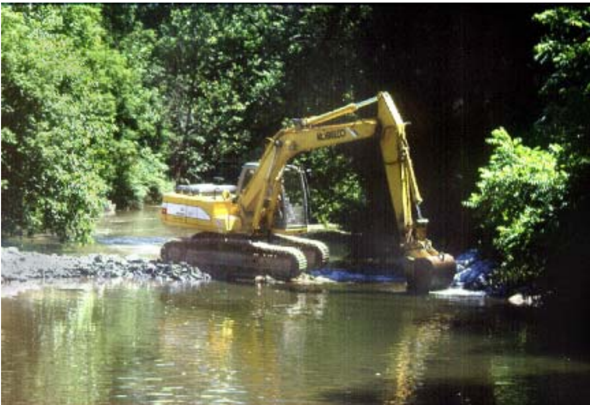
Figure 12. The opposite stream bank was stabilized with limestone riprap before the remainder of the dam was removed.
