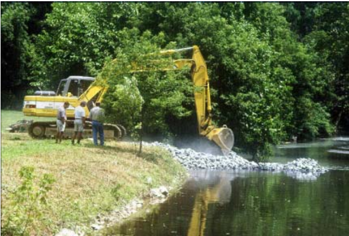
Figure 3. The equipment operator created a stone causeway to access the entire length of the concrete dam and a portion of the opposite streambank.
