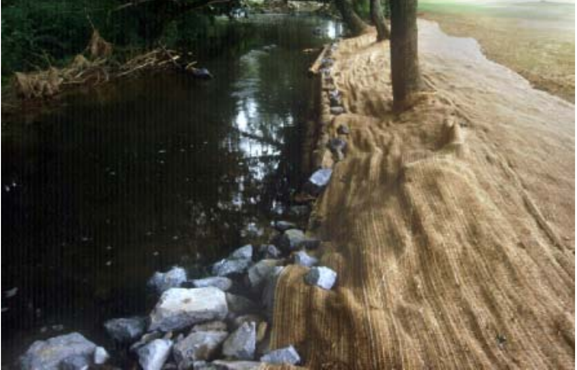
Figure 4 – Modified bank cribbing with seeded jute matting. Jute matting minimizes future soil erosion and provides moisture retention essential to the development of newly planted seed.
