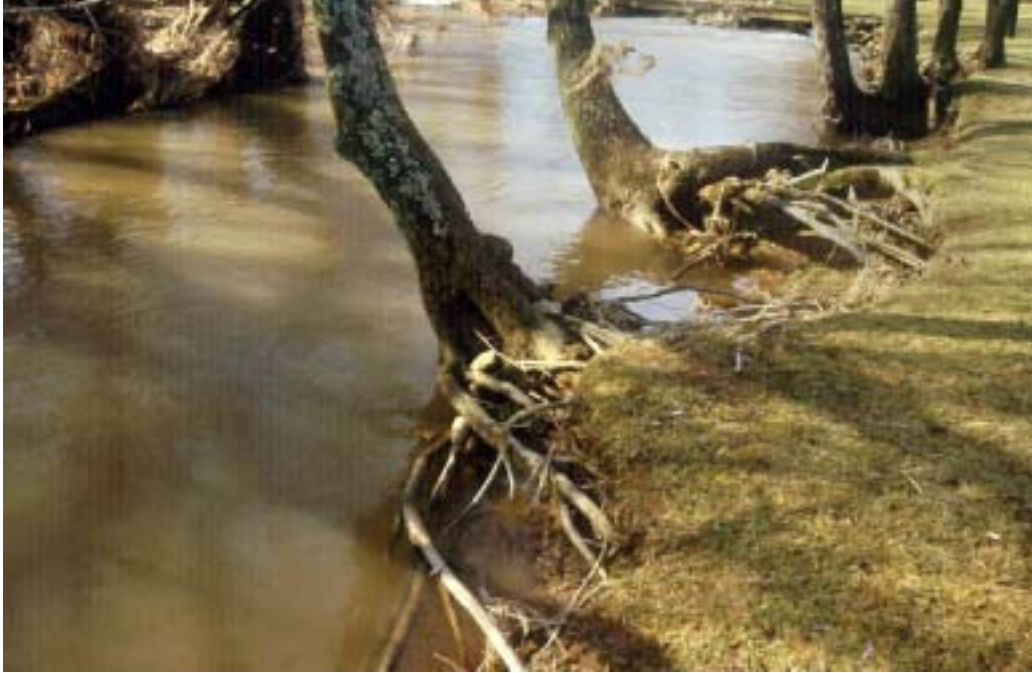
Figure 2 – Proposed site of modified bank cribbing. Note the severely eroded stream bank and lack of in-stream habitat.
