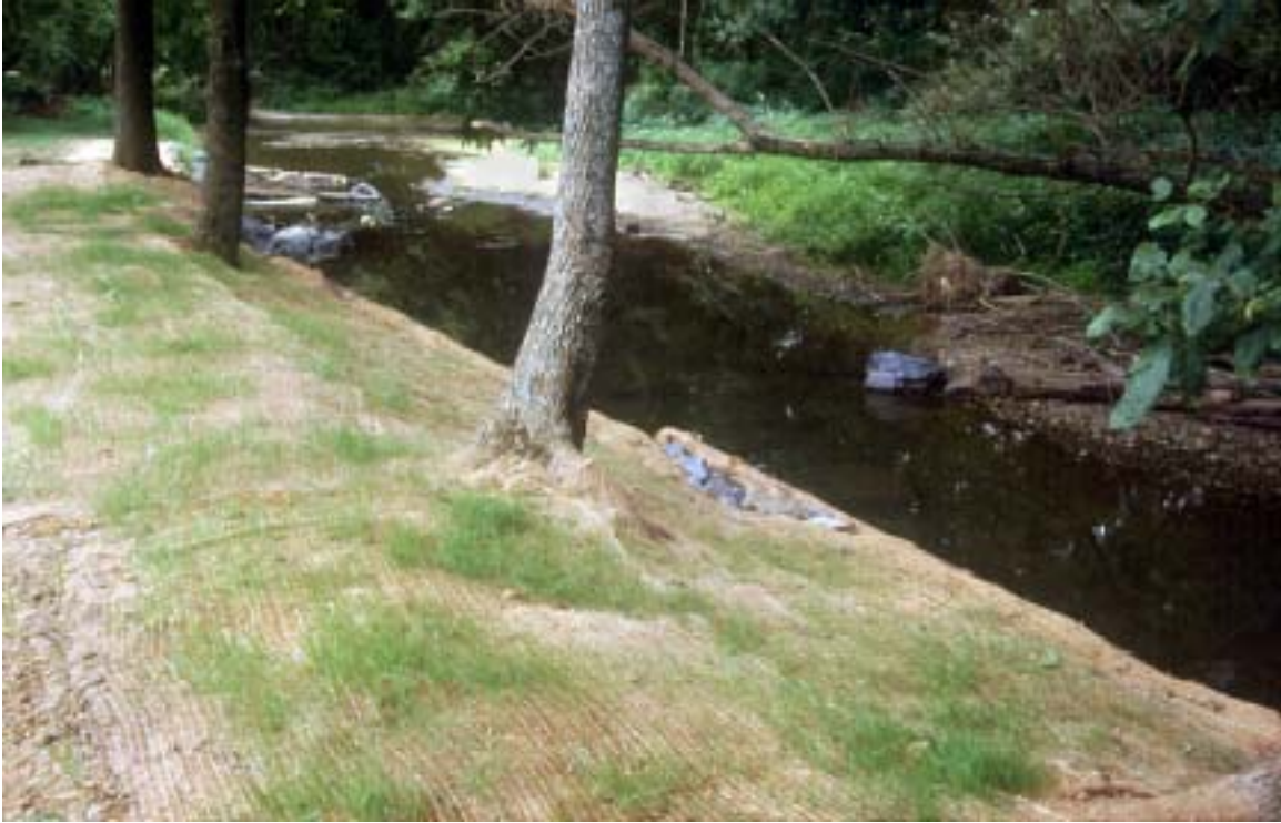
Figure 6 – Modified bank cribbing with seeded jute matting one month after construction. A stable undercut bank has been established. The grass will provide future stability to the stream banks during high flow.
