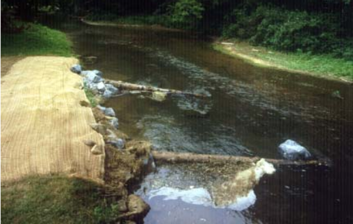
Figure 7 – Placement of upstream single logs deflects water from an eroded stream bank and provides naturalistic woody habitat for fish and aquatic macro-invertebrates. A scour pool will develop around the tips of the logs, offering overhead cover for fish.
